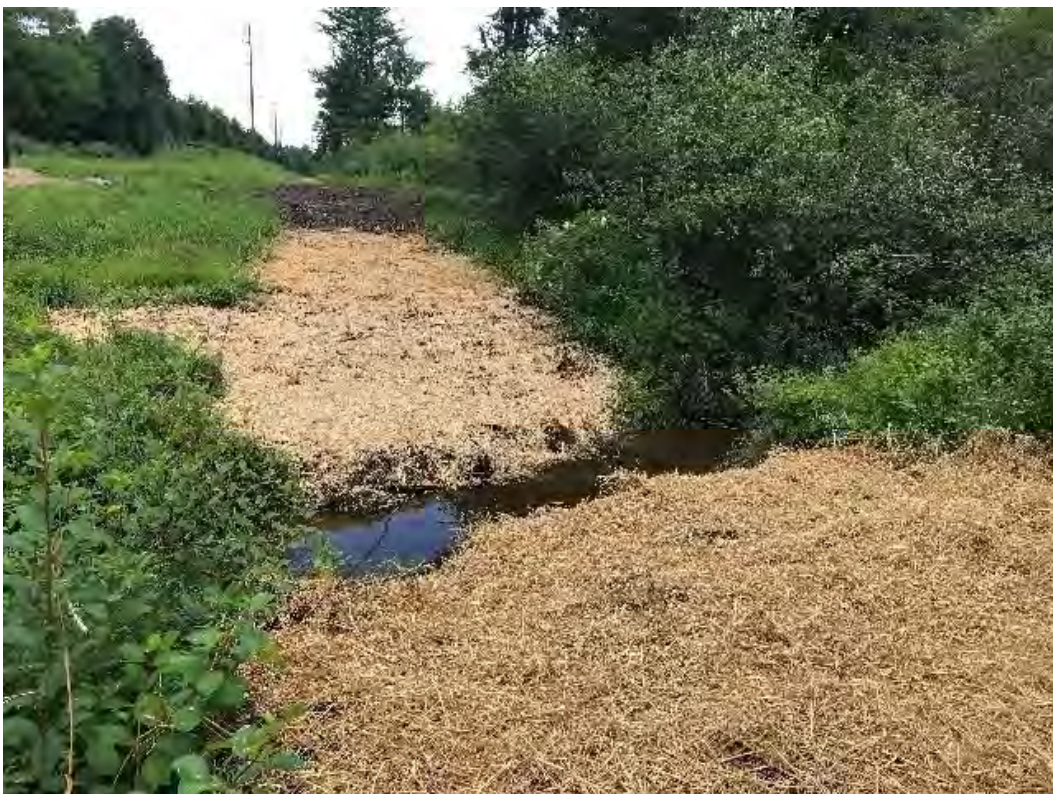
Fig 12: Restored access road and stream banks of stream DS60 between Strs. 44 and 45. Viewing north. (07-14-20).
