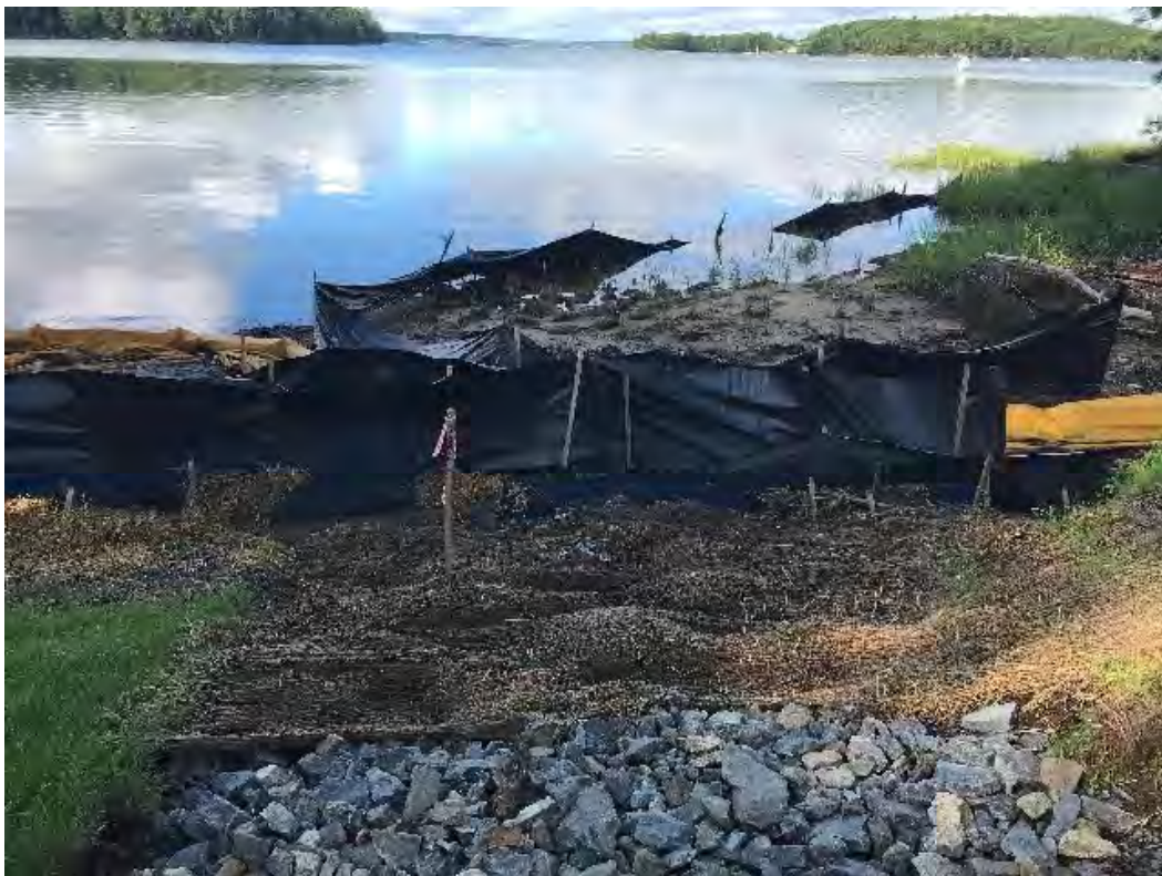
Fig 16: Temporary BMPs at toe of slope/intertidal zone at Gundalow Landing/east side of the bay. Viewing southwest. (07-15-20).
