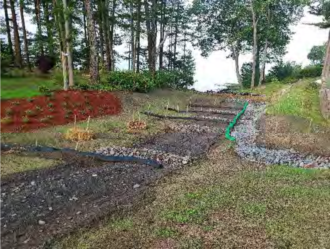
Fig 1: Temporary BMPs on slope above manhole at Gundalow Landing/east side of the bay. Viewing southwest. (07-09-20).
