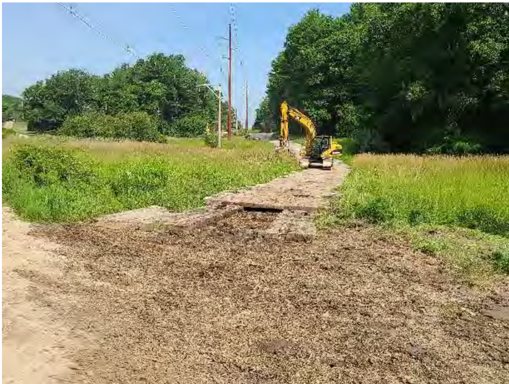
Fig 4: Removing timber matted access road in wetland DW6, between Strs. 95 and 96. Viewing northwest. (07-09-20).
