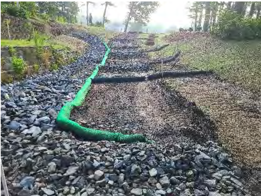
Fig 2: Temporary BMPs installed on slope above manhole at Gundalow Landing/east side of the Bay. Viewing west. (07-09-20).
